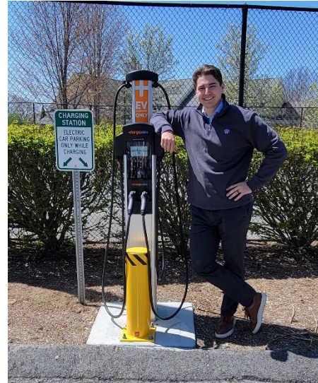
Dominik Kozlowski stands next to one of the EV Charging stations at Windsor Ridge Apartments in Westborough
